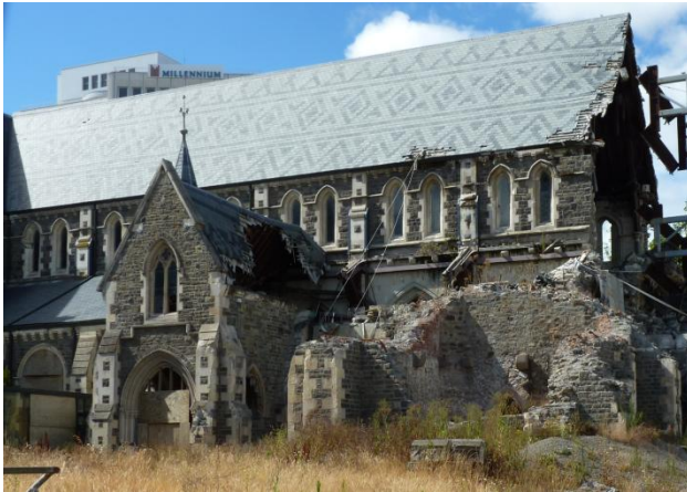
A badly damaged Christchurch Cathedral
